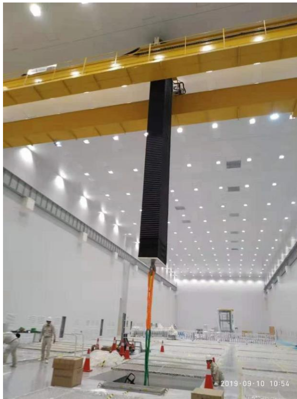
Double girder Clean room crane
