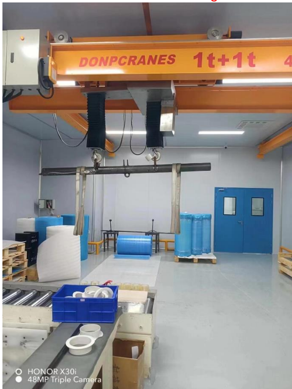
Single girder Clean room crane
